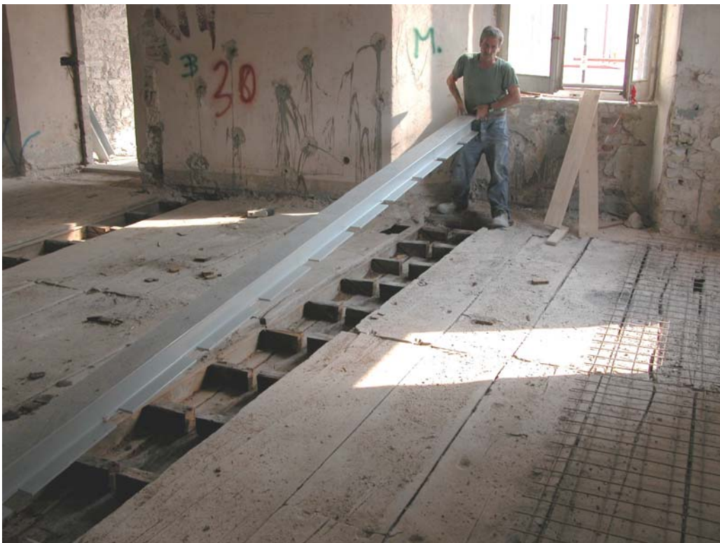
Figure 9-4 –Strengthening intervention on the main beams (Designers: ingg. A. Giannantoni e F. Menghini, in collaboration with prof. A. Borri).
